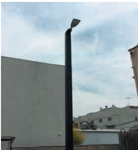
USA – Asima® Sun, Standalone, and Monopole, Standalone, In cooperation with Los Angeles Municipality
